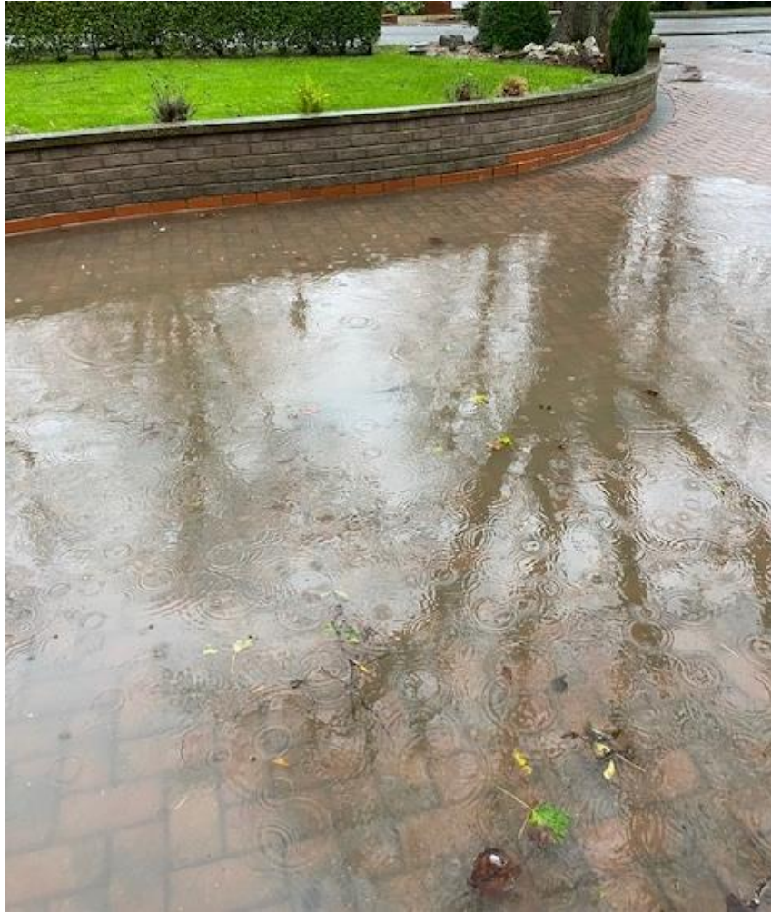
(Figure 12 – Flooding in the front driveway at Property C, as provided by the resident; facing south)
