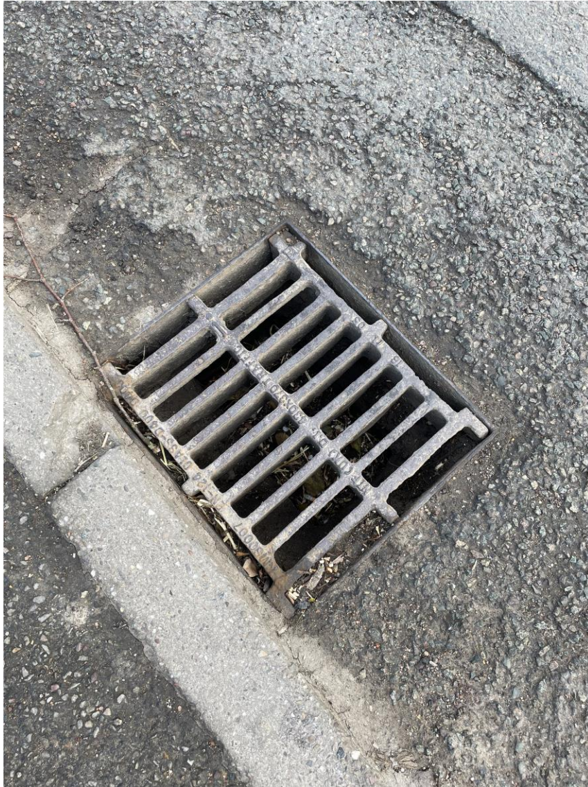
(Photograph 7 – Gully outside Property D, which appeared to be partially blocked with silt and plant debris)
