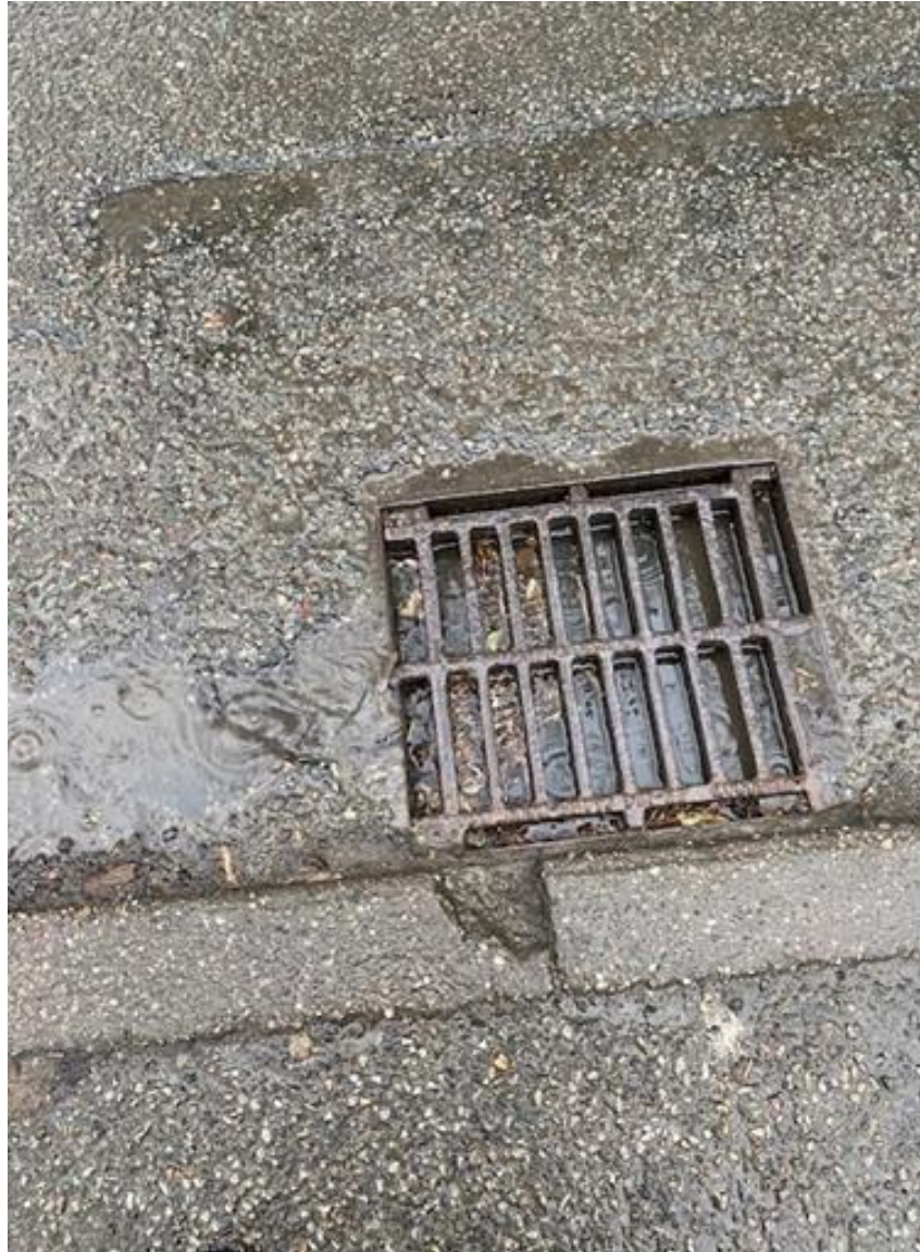
(Photograph 9 – Gully outside Property D at full capacity during 15 th of April, indicating potential blockage)
