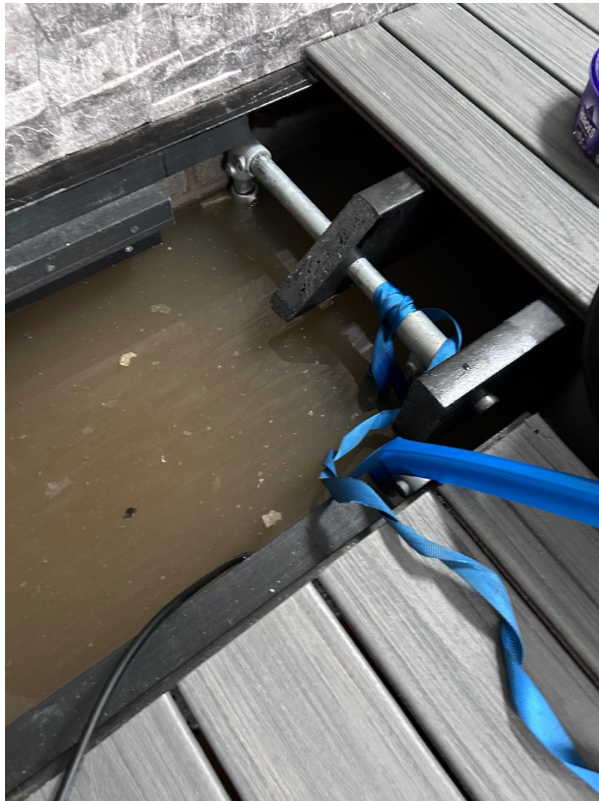
(Figure 17 – Flooding beneath the floorboards in the extension at Property D, as provided with the resident)
